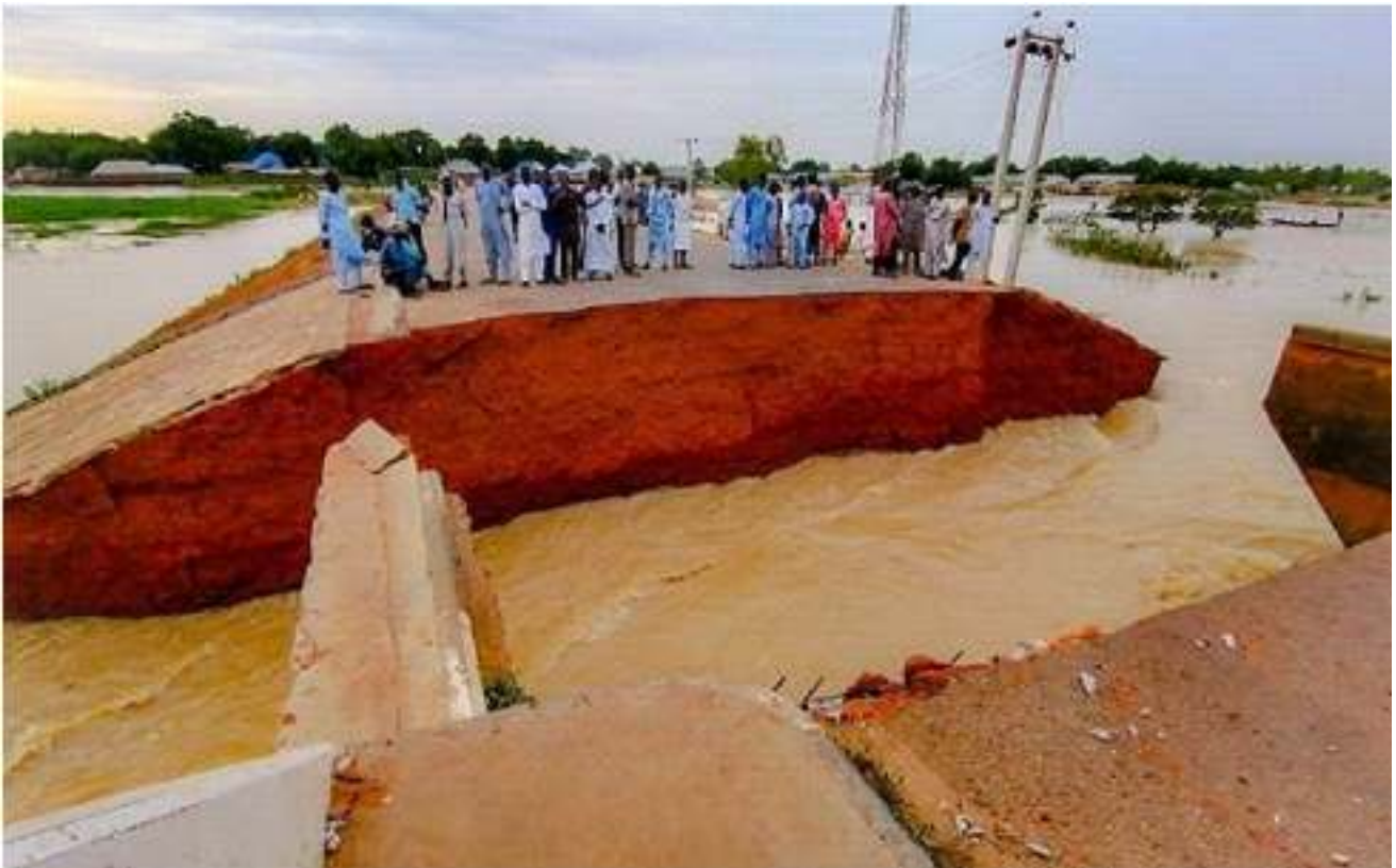
Figure 1.8: Submerged Bridge due to flood effect in Kebbi State.
