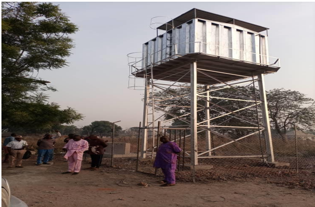
Motorised Solar Powered Borehole at Stepen Machi Compound Ningeve, Vandeikya LGA, Benue State
