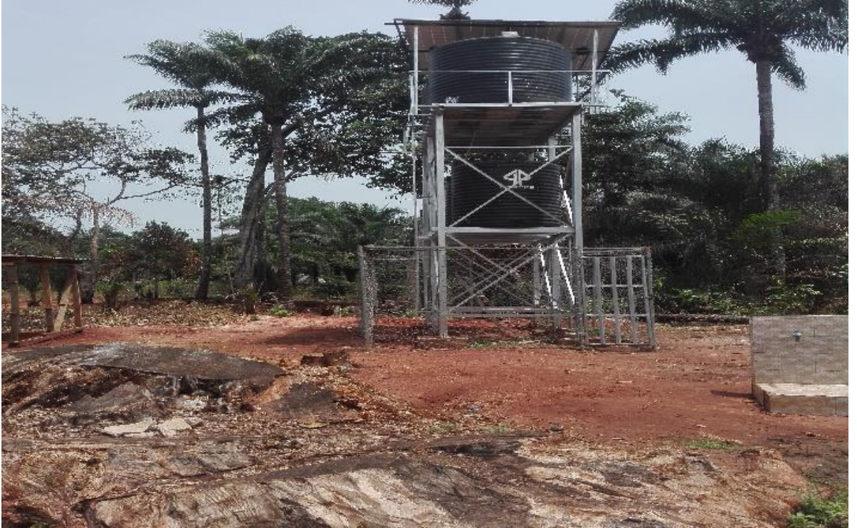
Solar Powered Borehole with 1km Reticulation at Aguneze Ahiazu Mbaise, Imo State
