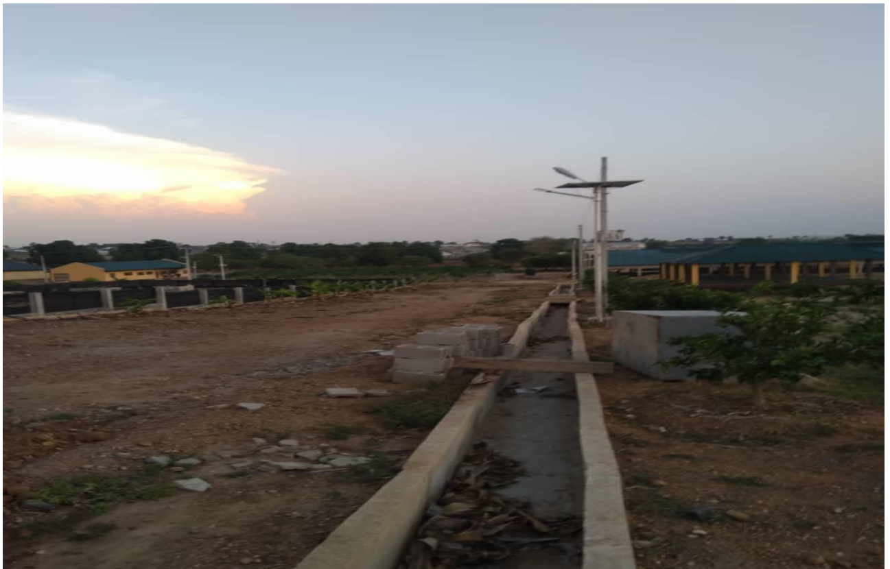
Enhancing Irrigation Potential in FCT through Land Clearing and dredging of waterways (dredging at Gada-Biyu Irrigation Project Kwali Area Council)
