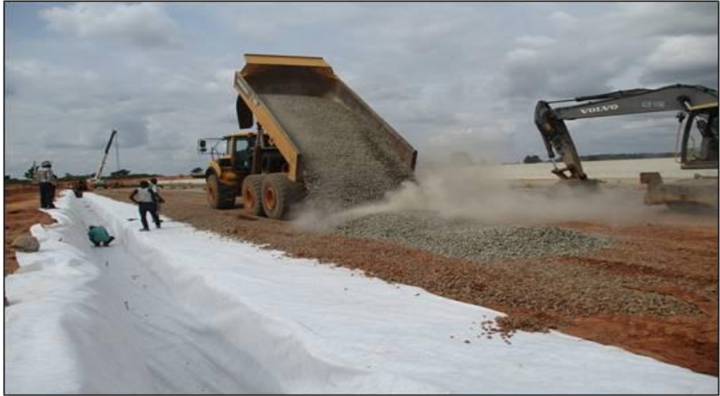
Laying of Geotextile and Chippings in Toe Beam Trench and floor of Step no. 4
