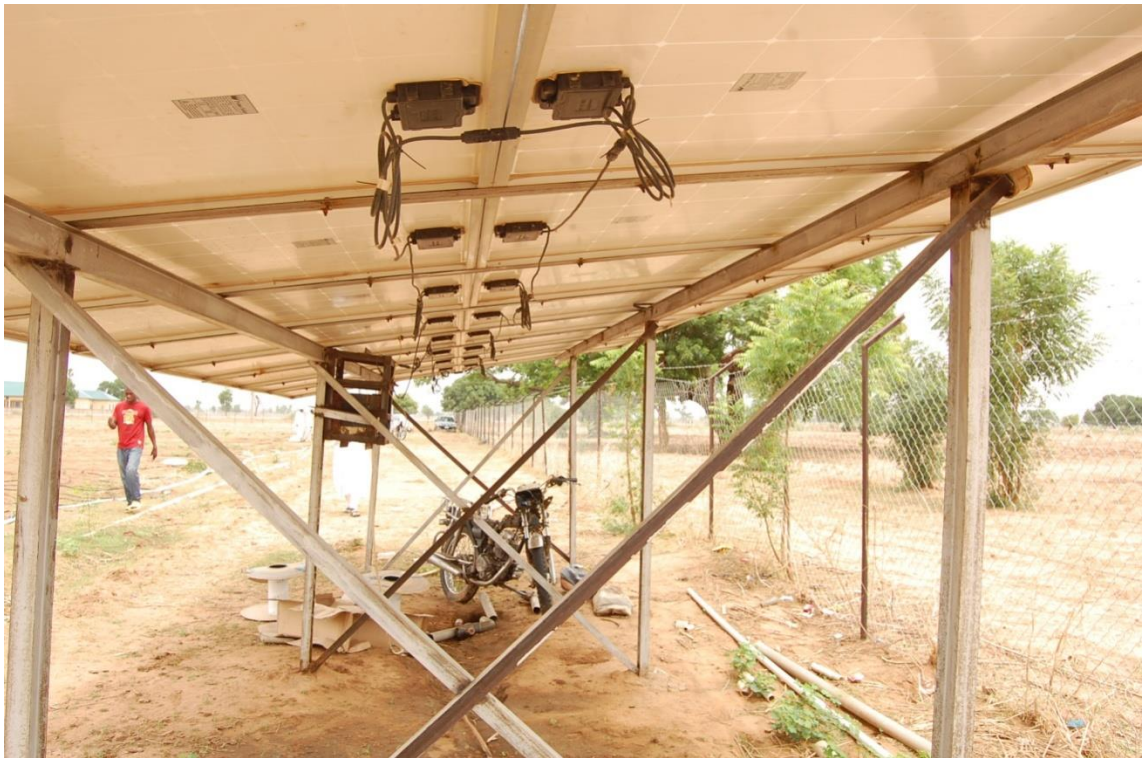
Installation of Solar Powered Pump Based Drip Irrigation at Sawe Pilot Irrigation Scheme, Bauchi State in progress
